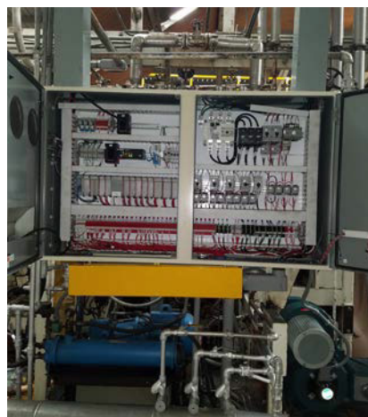
New PLC Remote I/O and Controls —Machine Mounted
