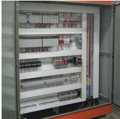
Allen-Bradley ControlLogix PLC
